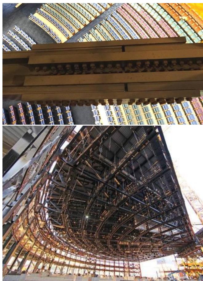
Figure 3-7. Bolted connection - Epic, Deep Space Auditorium in Verona, Wisconsin (credits Robert Caroti/ArcelorMittal International and Vakaris Renetskis).
